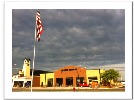
Progress being made on the City of Boyne City's new complex which will house the new BCFD. Picture taken June 3, 2017.
