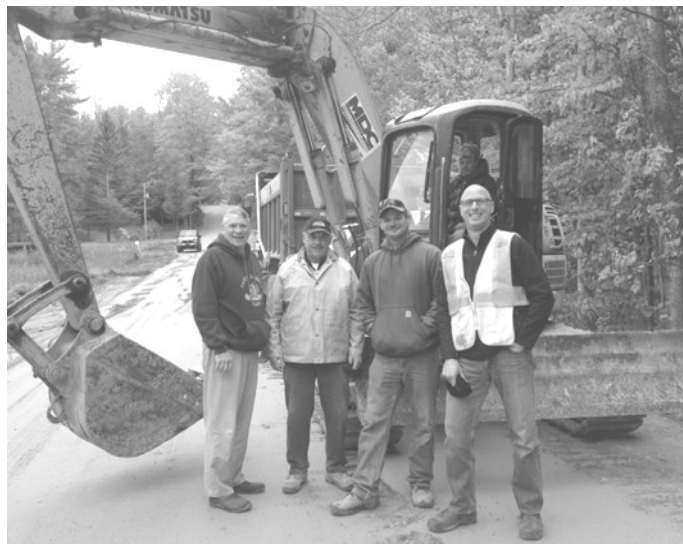
Observing the excavation and paving of Church Road are (from left): Bill Wehrenberg, Township Trustee, Gary Leist and James Schillinger of MDC Contracting, Jim Vanek, Township Clerk and the Engineer for the Charlevoix County Road Commission, and Ron Goff, MDC Contracting (sitting in the excavator). (photo courtesy of Jane Wehrenberg)
